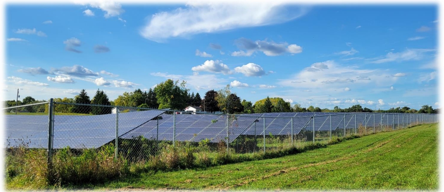
Onsted Schools Solar Project
